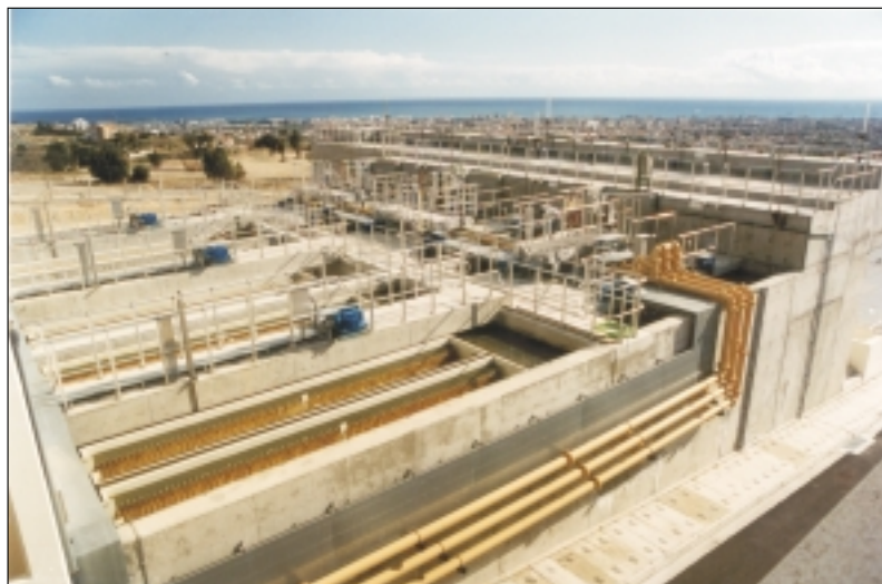
Limassol Water Treatment Plant
