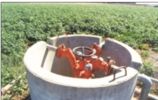
Hydrant with three outlets
